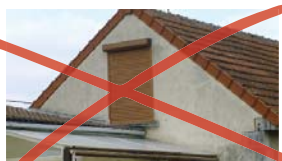
Percements proche pignon
